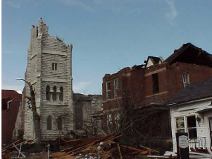
Figure 2. Damage to historic downtown church (photo downloaded from NOAA web site at http://www.srh.noaa.gov/ohx/?n=stormsurvey01221999 )
