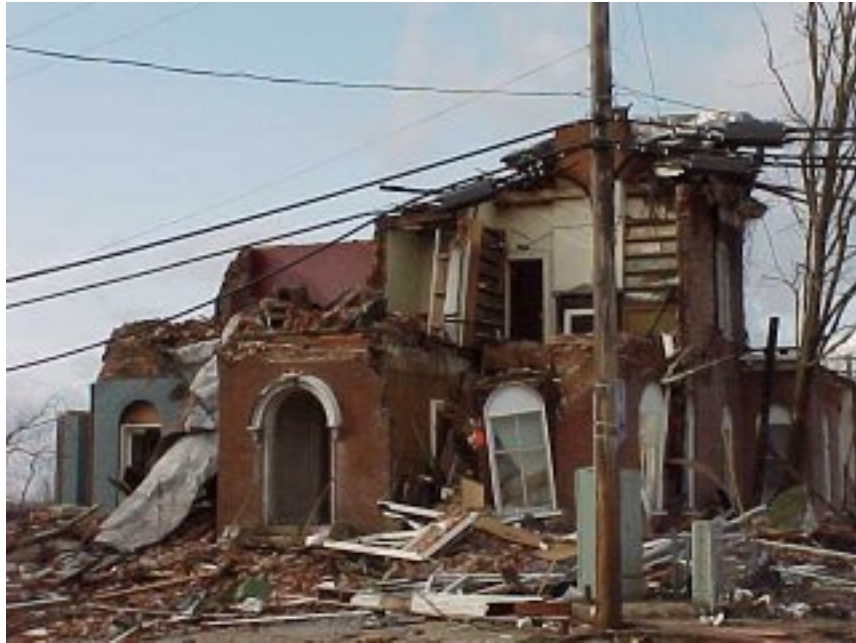
Figure 3. Damage to historic downtown residence (photo downloaded from NOAA website at http://www.srh.noaa.gov/ohx/?n=stormsurvey01221999 )
